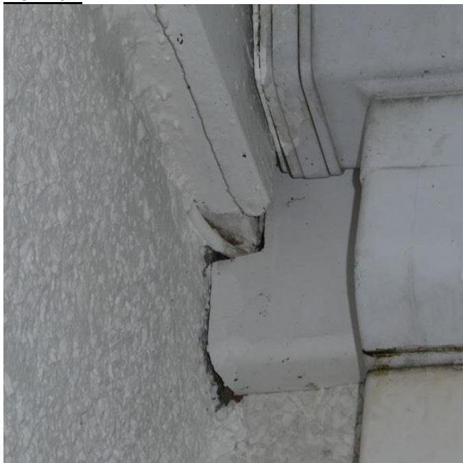
Unsealed And Open Facia Abutment Joint To Wall
