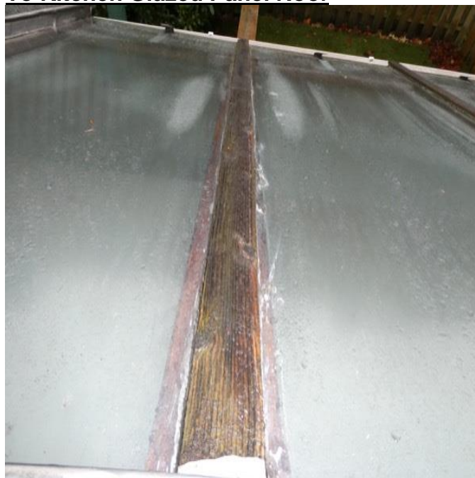
Exposed Timber Roof Bar Joints Detected To Kitchen Glazed Panel Roof
