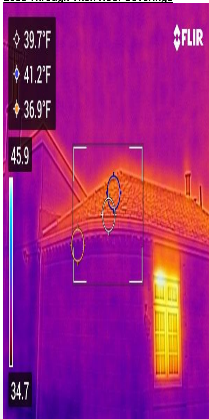
Thermal Image Shows High Levels Of Heat Loss Through Then Roof Coverings
