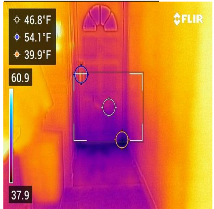
High Levels Of Air Filtration Detected To The Base Of The Door Threshold
