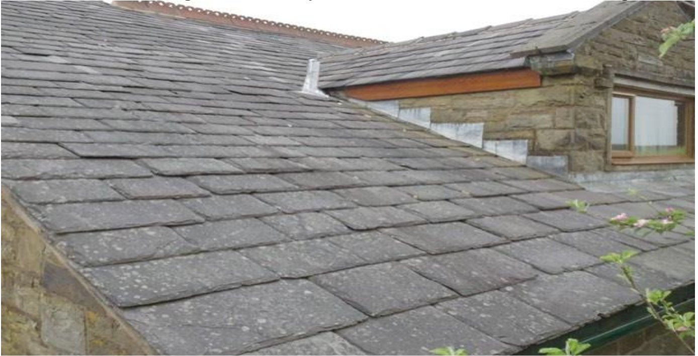
View of the roof covering to the two story addition at the front of the main building.
